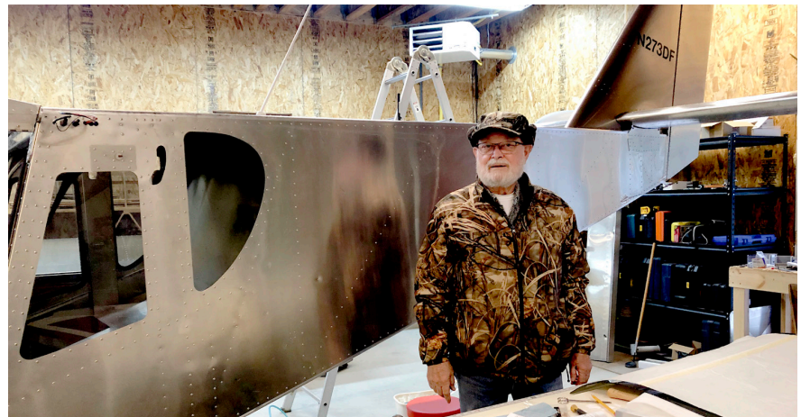
Don pictured with the tail section of the 820 lb. plane. Speed is 100 MPH. Don had a immense repair job, but today the plane is flying again.
